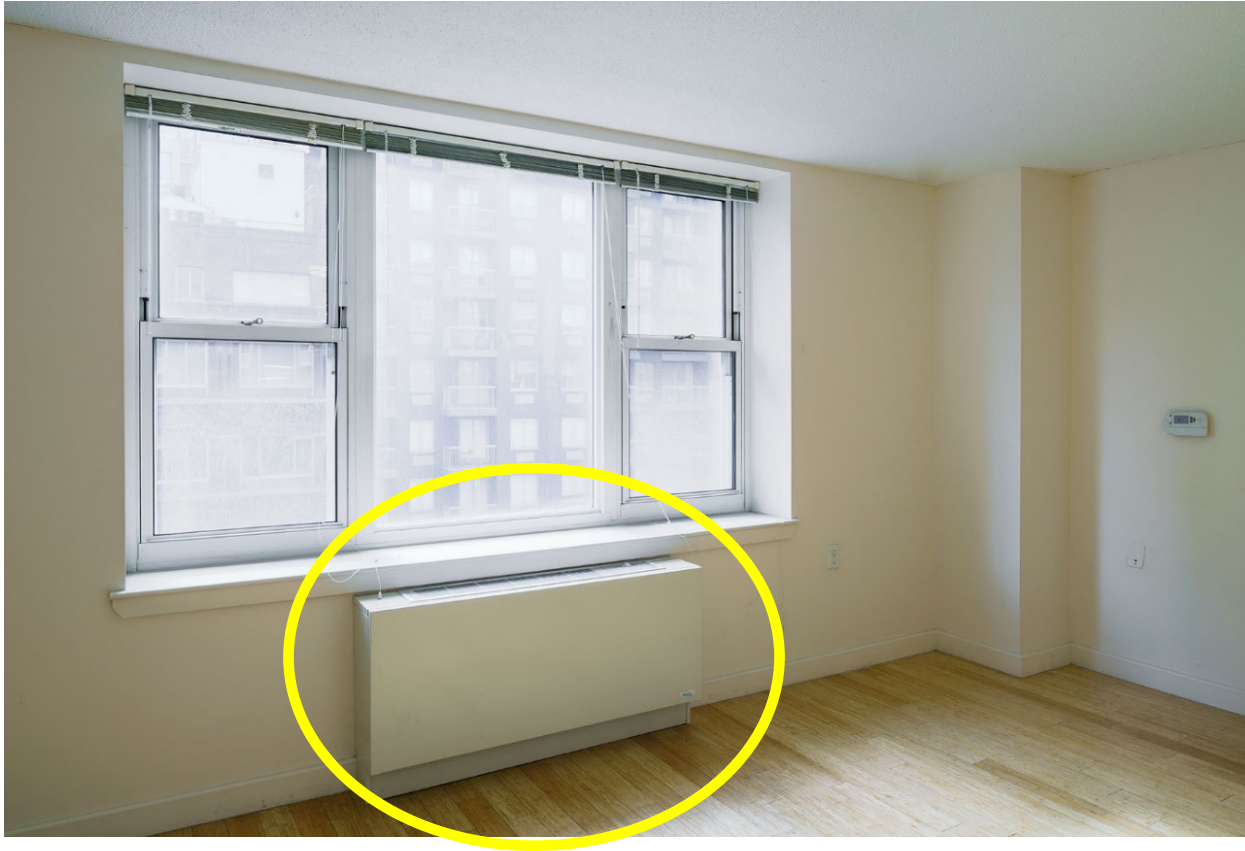
Condenser in existing sleeve + evaporator on wall
